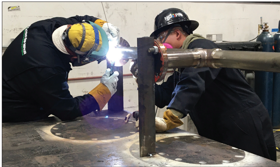
Julius Agahan welds a section of pipe to be installed in an aircraft carrier in STANDARD’s Barrio Logan shop. Helping on the right is Patrick Caniya . Photo by Brad Graves
